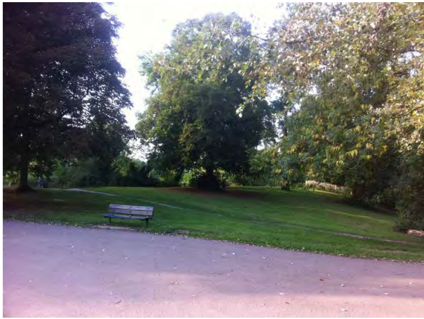
View North on down stream slope of dam at Highgate No.1 Pond Existing
